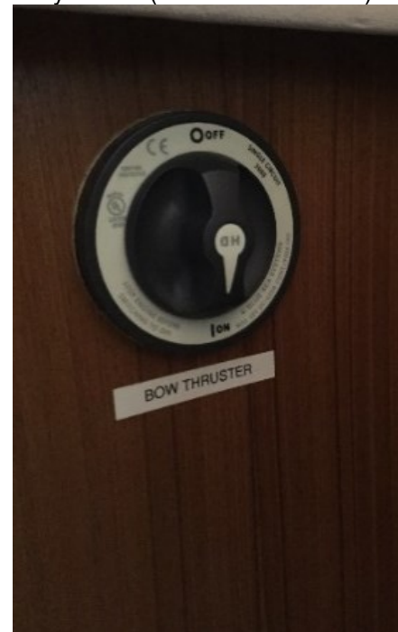
Bow Thruster Battery Switch (Forward Stateroom)
