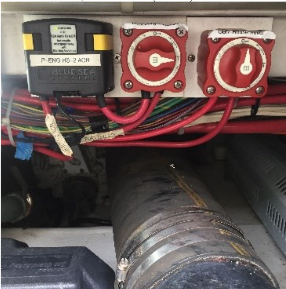
Port Alternator X-over, Generator X-over (Lazarette)
