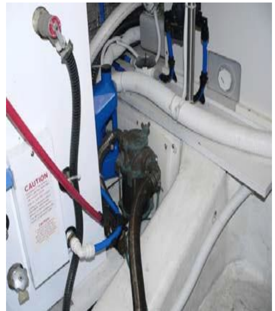
The genset sea strainer, with its through-hull right next to it, forward in the engine room.
