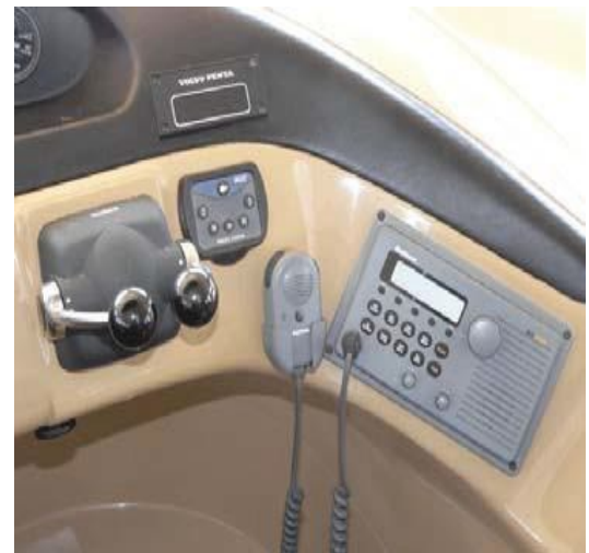
The VHF radios are beside each helm station. This is the pilothouse unit.
