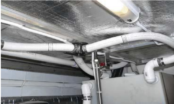
Y-Valve on ceiling of Engine Room port forward. Switch for overboard pump (red).
