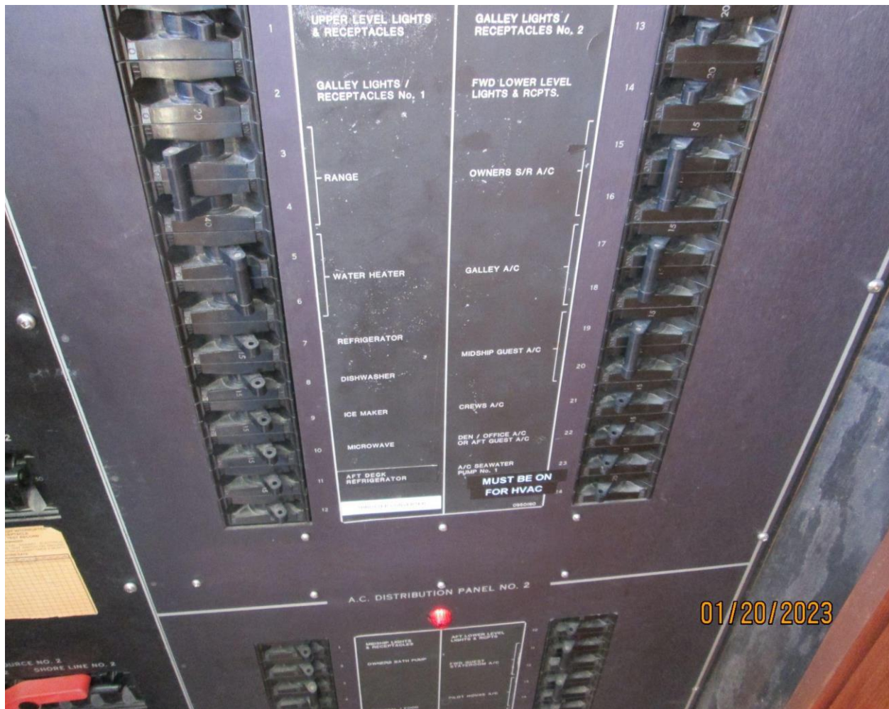
OCEAN ROMANCE ELECTRICAL PANEL
