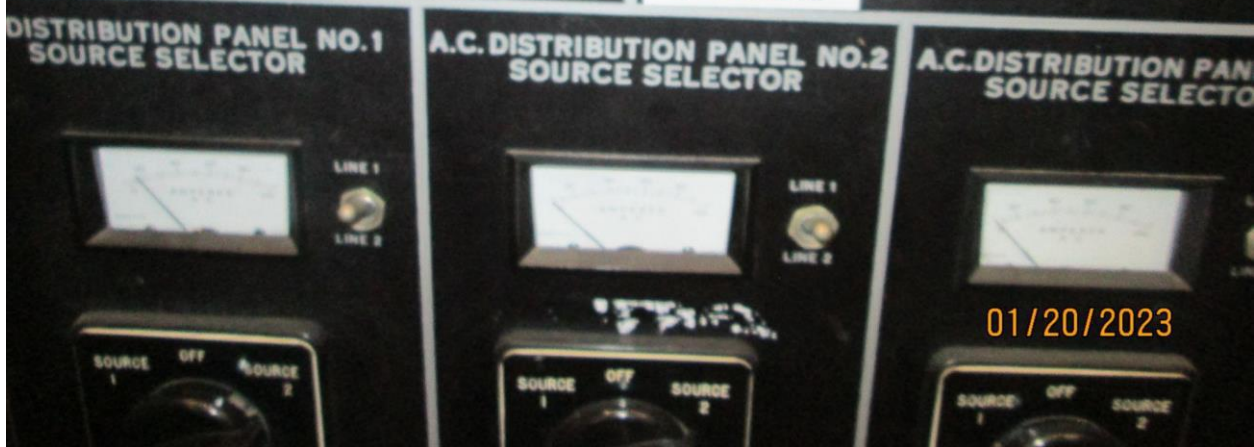
OCEAN ROMANCE ELECTRICAL PANELS
