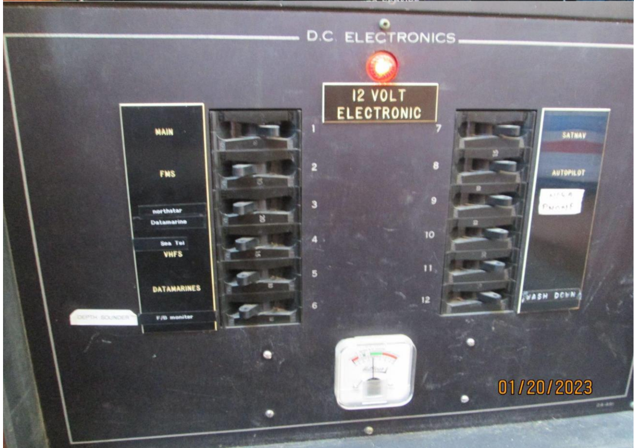
OCEAN ROMANCE ELECTRICAL PANELS
