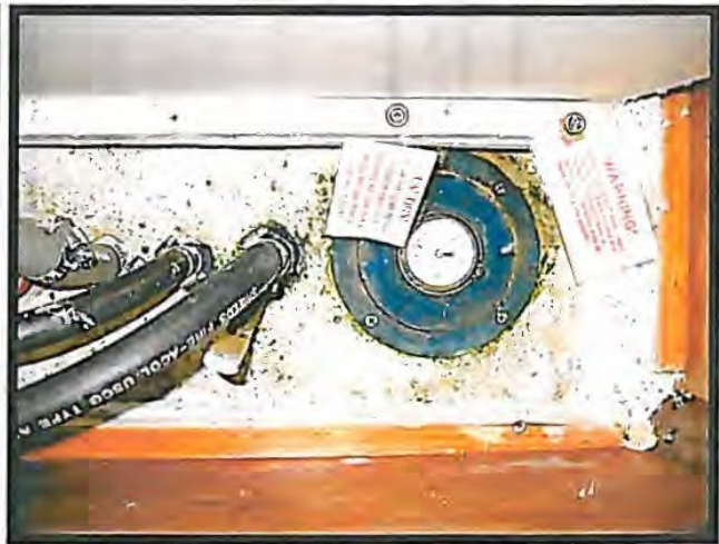
Fuel Tank Gauge Under Port Salon Seat
