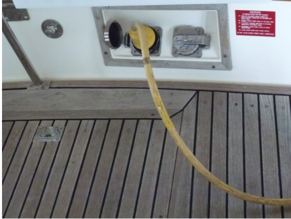
AFT SHORE POWER CONNECTION
