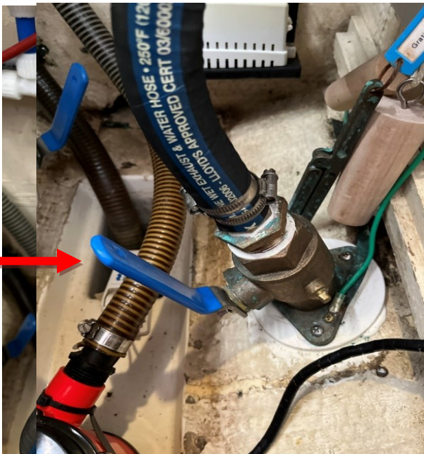
RAW WATER INTAKES
