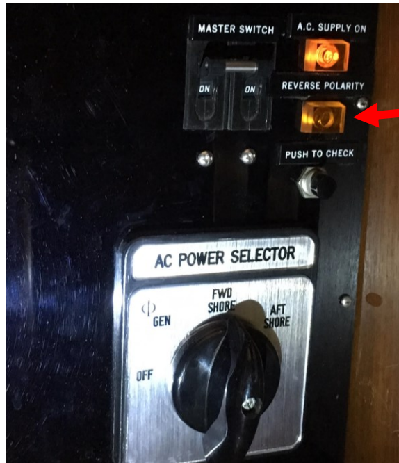
AC POWER PANEL
