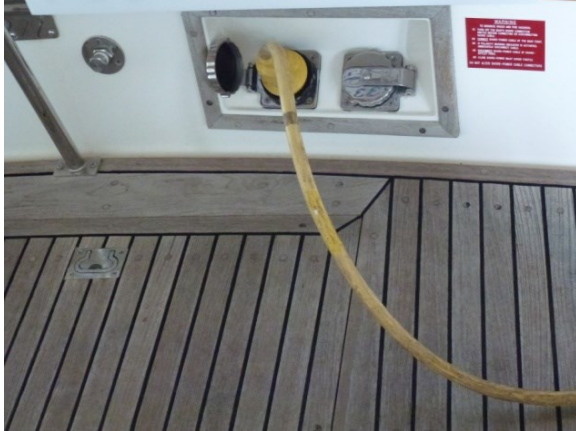
AFT SHORE POWER CONNECTION
