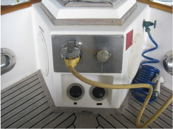
FORWARD SHORE POWER CONNECTION
