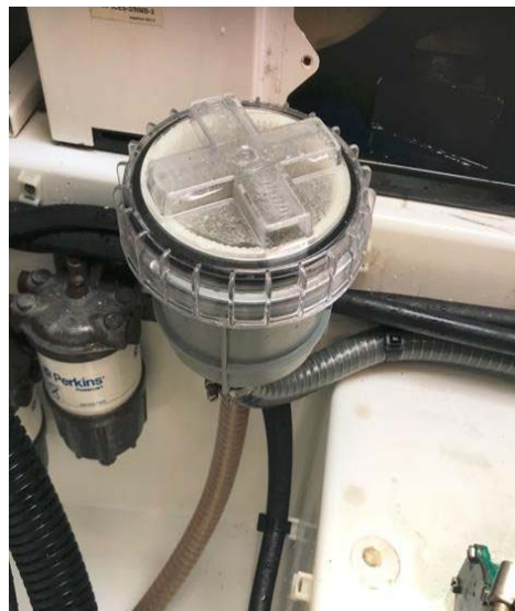
Generator raw water strainer located in port engine room.
