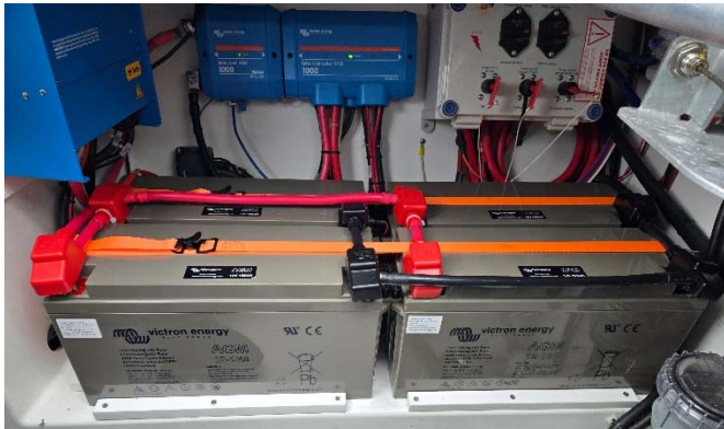
House bank. Stbd Engine Comp
