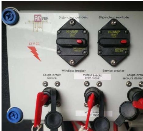
Emergency parallel switch
