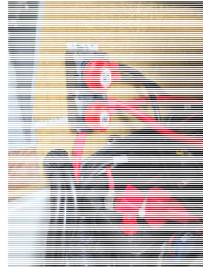
Genset & Port Eng Start Batteries
