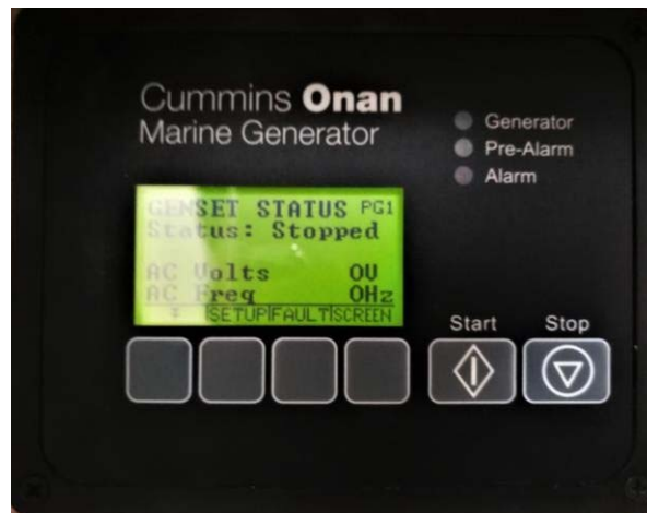
Generator control panel in salon
