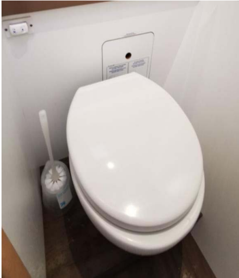
Starboard Holding tank seacock
