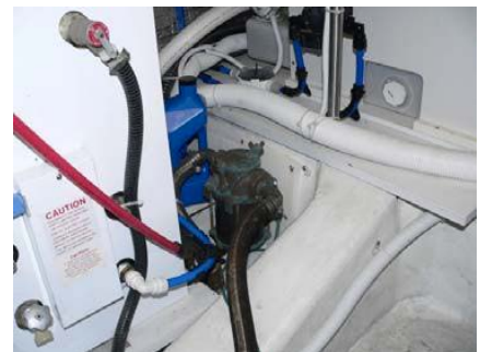
The genset sea strainer, with its through-hull right next to it, forward in the engine room.
