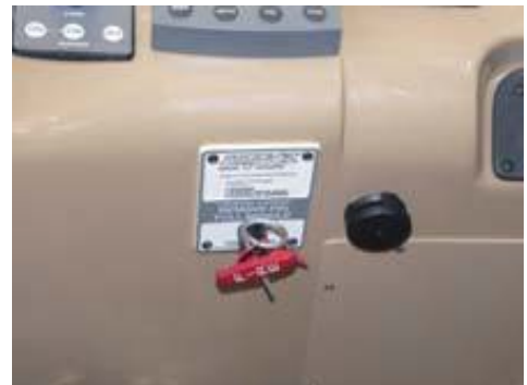
Engine Room Fire Extinguisher emergency control is located on the lower helm. Pull pin and then pull handle to activate.
