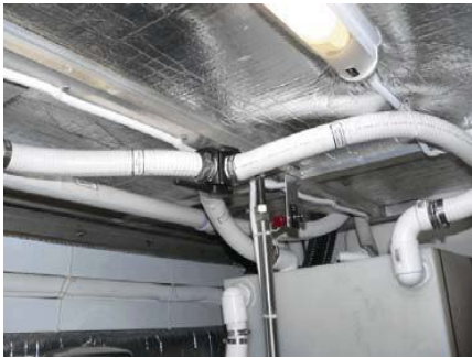
Y-Valve on ceiling of Engine Room port forward. Switch for overboard pump (red).
