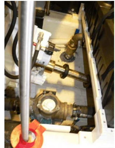
Port main engine sea strainer in foreground; its valve is just on the far side of shaft, with blue handle on far side “up”/open.
