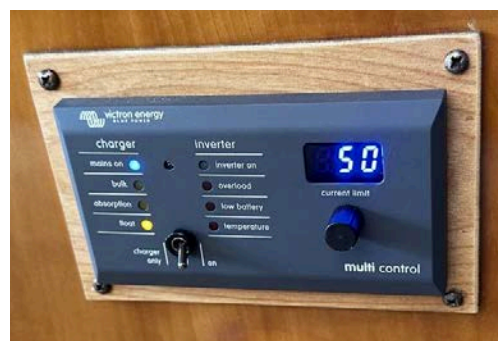
Inverter control panel by DC panel.
