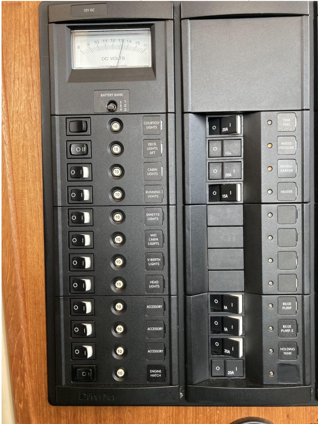
House DC Panel (located behind salon settee)
