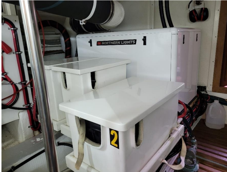
The location of the Northern Lights generator is aft engine room on the starboard side. Note sea strainer at bottom right of image.
