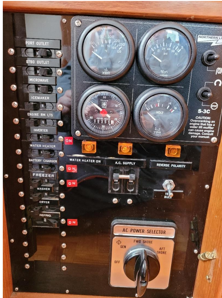
AC 110 Volt system, generator control and AC power selector.
