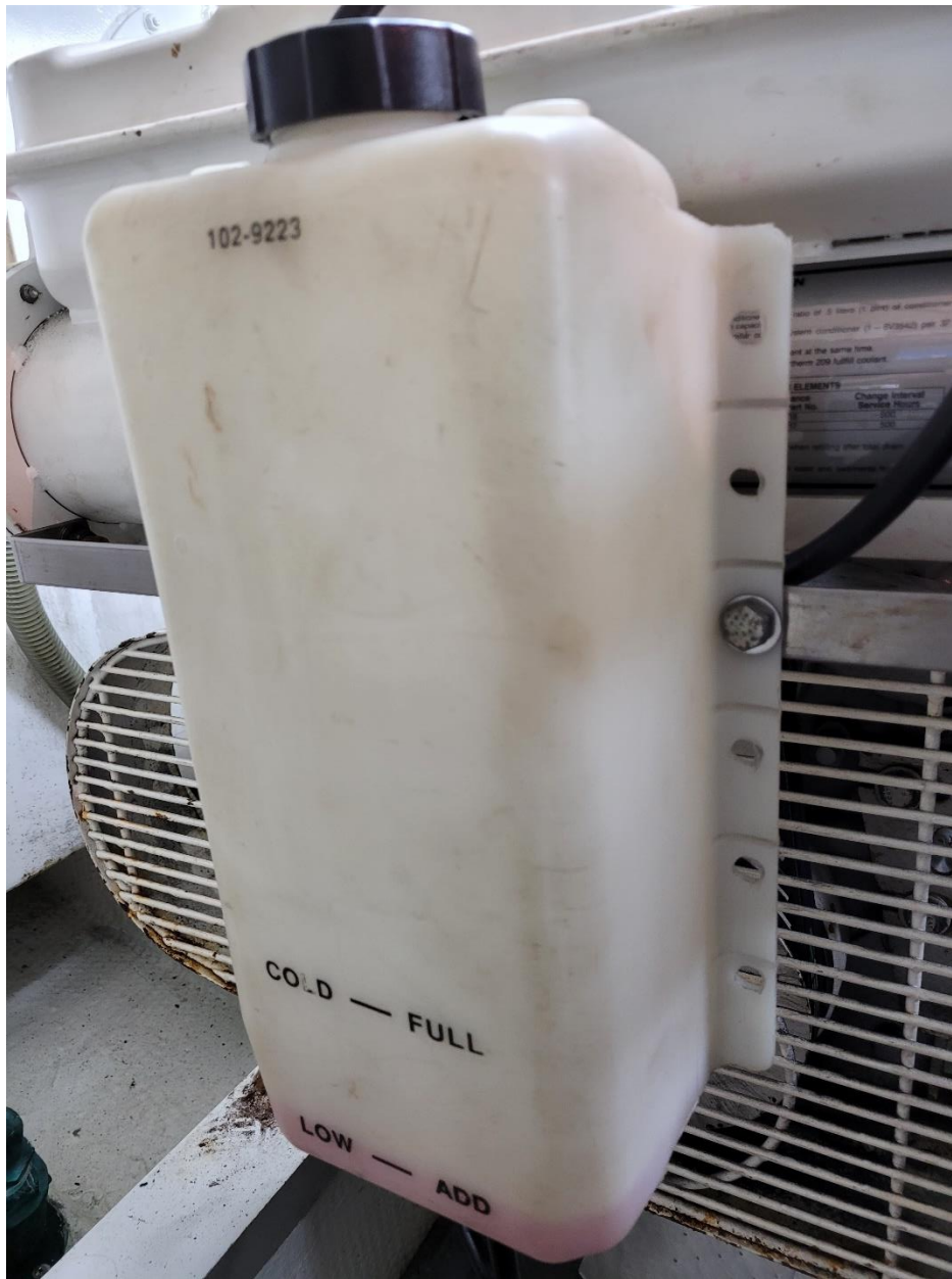
Starboard engine coolant reservoir Note: FULL line when cold, do not fill above this.
