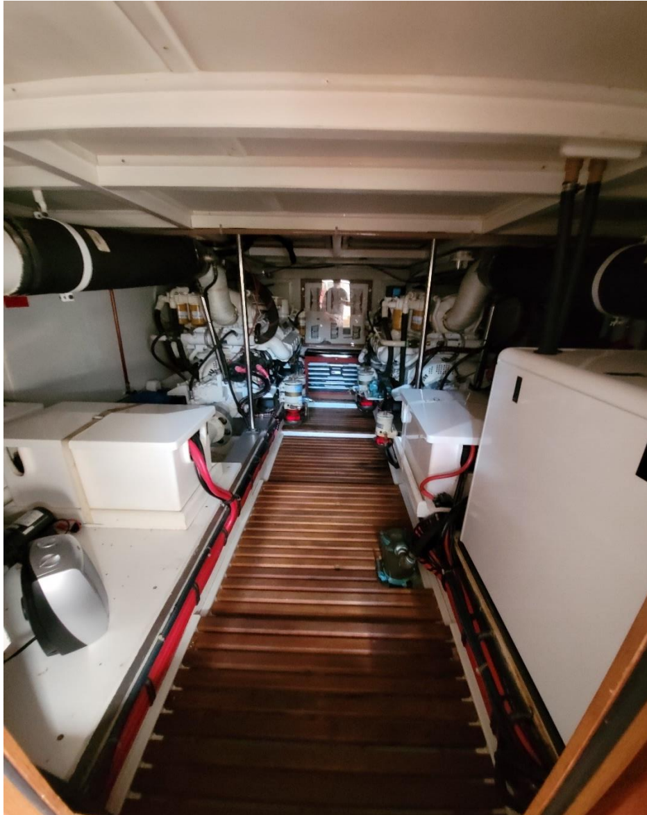
Engine room view aft to forward
