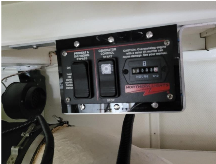
Generator local start and hour meter
