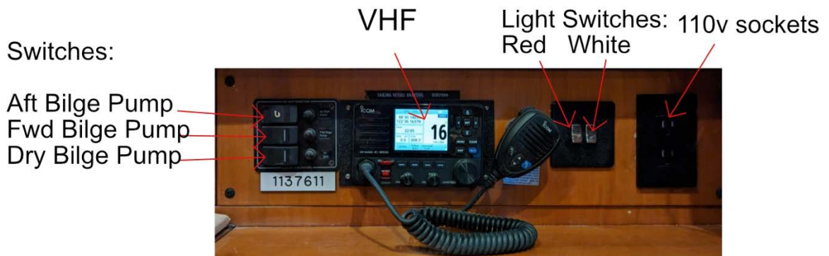
Figure 5: Navigation Station Lower Forward Panel
