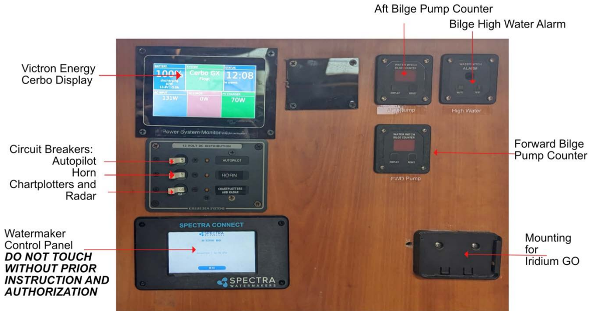
Figure 15: Secondary Power Control Panel
