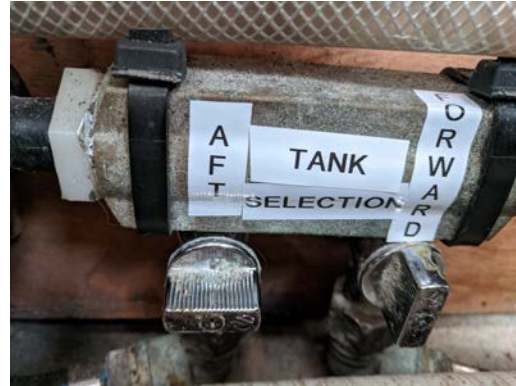
Valves set to draw water from forward tank.
