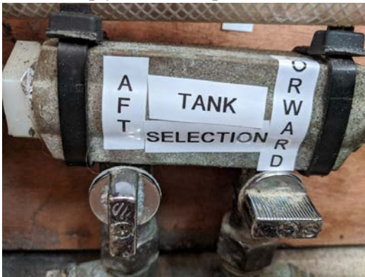
Valves set to draw water from aft tank.
